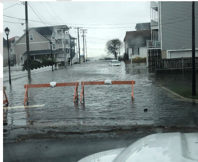
Photo 20 – Flooding along 9 th due to Inadequate Drainage
