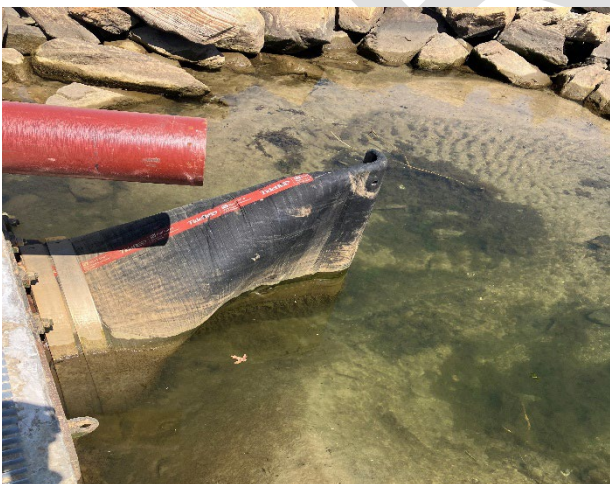
Photo 14 - New 5th Street Pump Station Duckbill Valve
