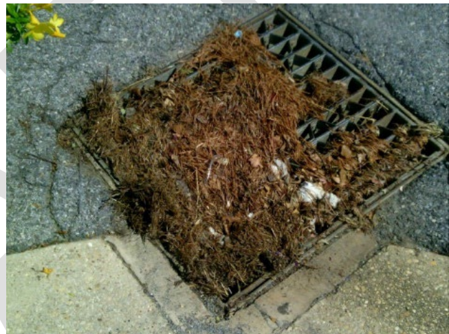
Photo 13 - Inlet Clogged with Debris
